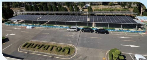
▲ Expansion of solar panels in the parking lot of the Yanshin Plant
